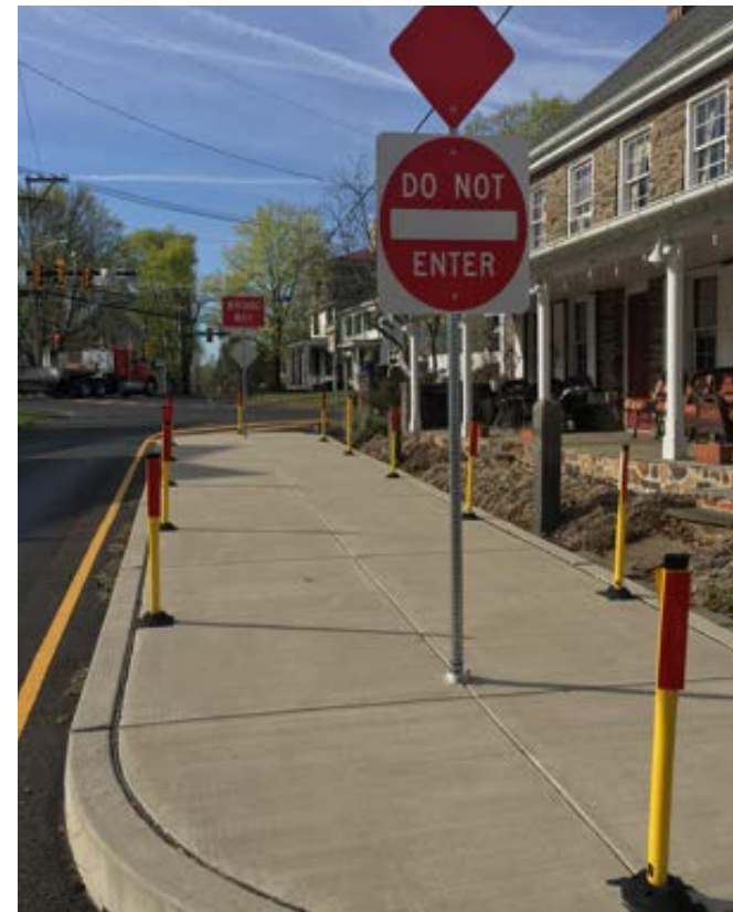
Concrete traffic island installed to block lane for one-way traffic on Old Skippack Road
